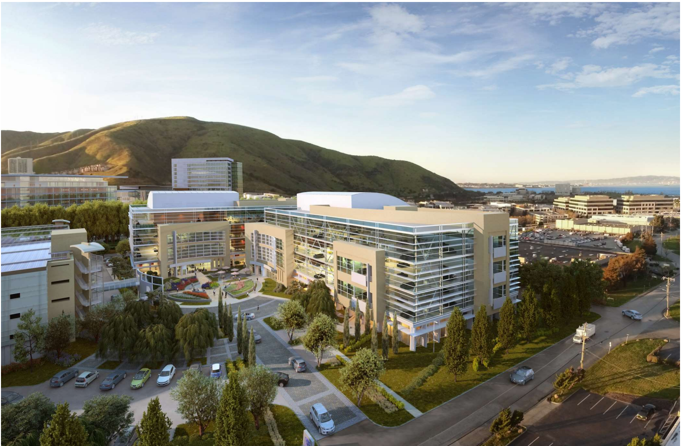
Construction on Gateway of Pacific's fourth phase is underway and will add another roughly 320,000 square feet to the campus' expanse. (CoStar)
