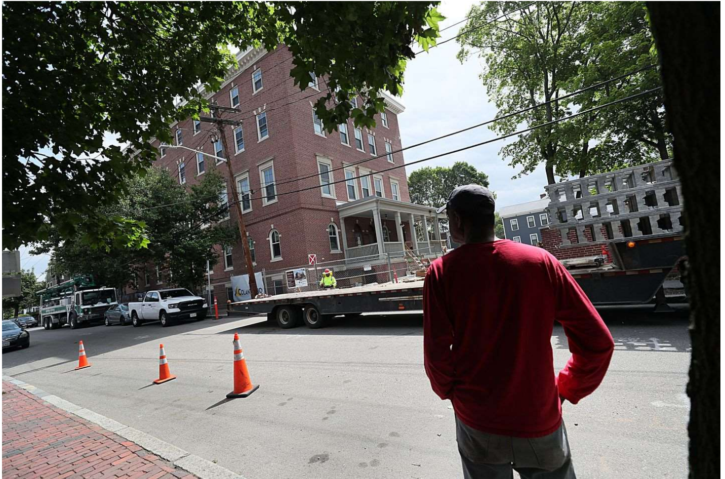
Construction at 116 Norfolk St., a public housing development near Central Square. SUZANNE KREITER/GLOBE STAFF
