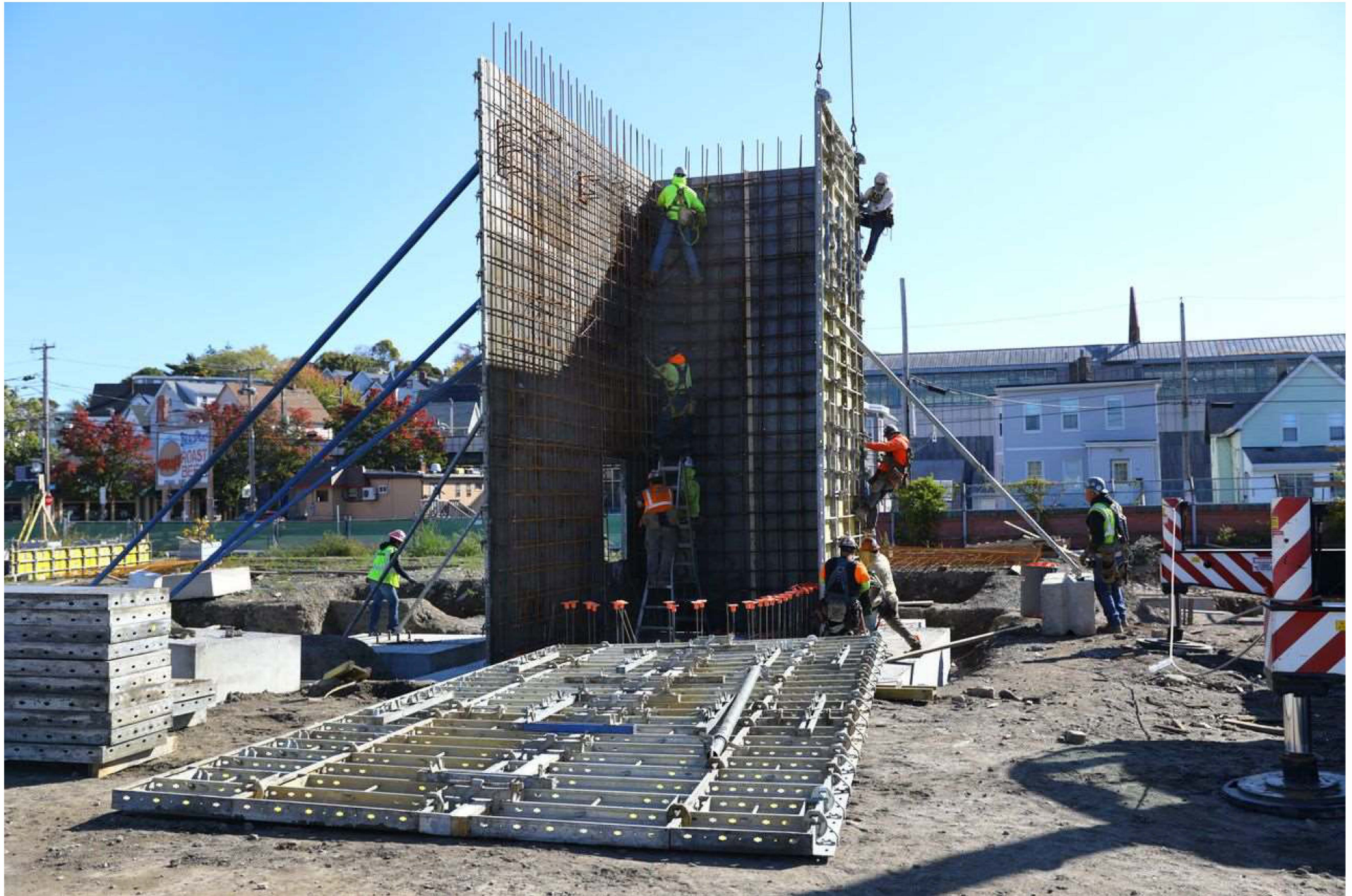
Construction of an apartment complex is underway on the Suffolk Downs site in Revere on Oct. 20, 2022. PAT GREENHOUSE/GLOBE STAFF
