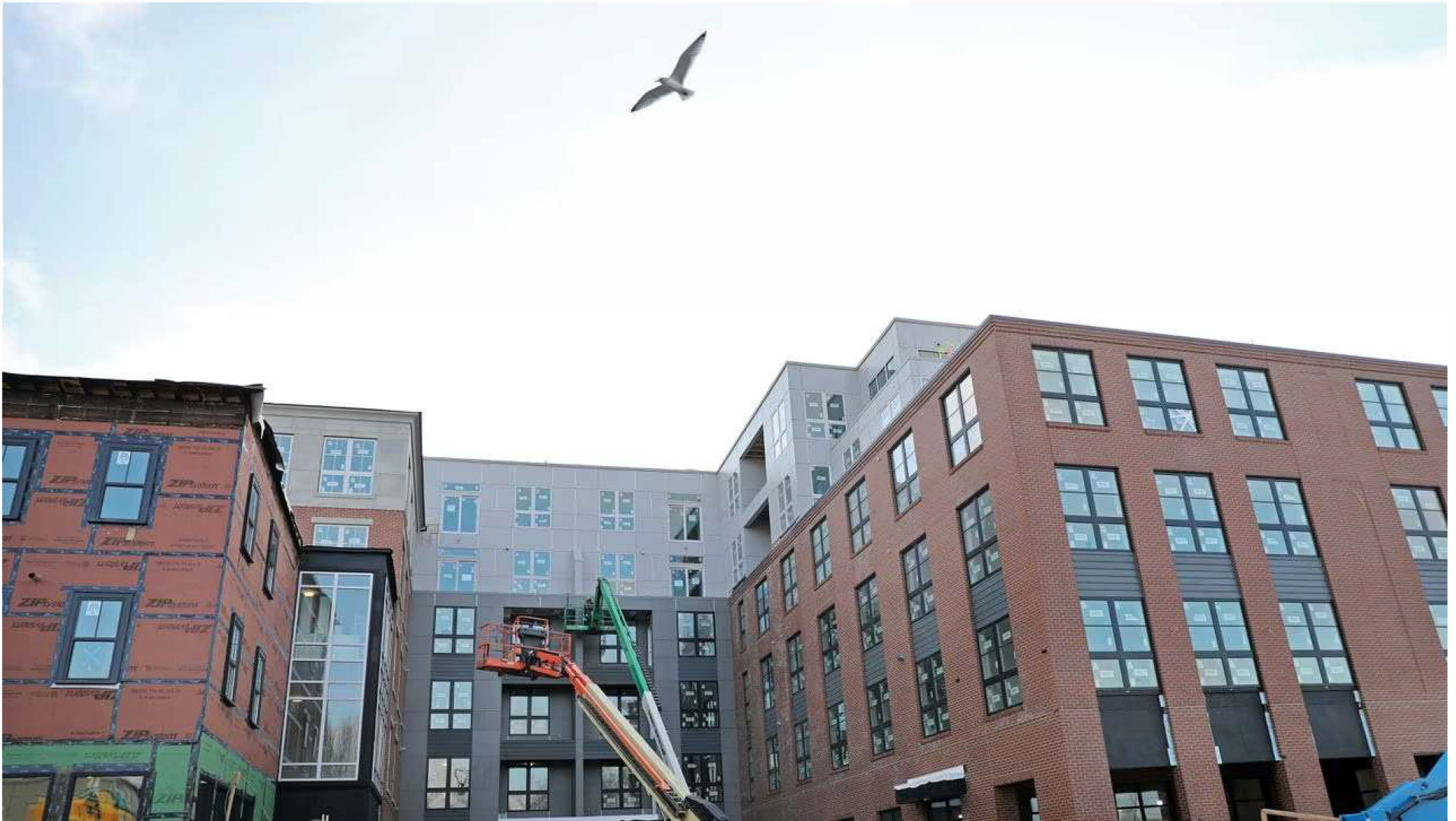
Construction at Rantoul Street and Railroad Avenue in Beverly on Jan. 11, 2023. PAT GREENHOUSE/GLOBE STAFF
